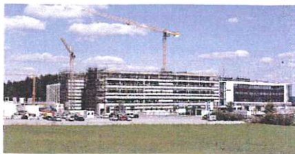
Structural work for the expansion at Ravensburg Vetter West is complete; the site will be operational by 2017
